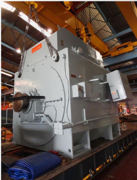
Extensive repair work was undertaken by M&C on a 28 MW synchronous motor for Saldanha Steel.
