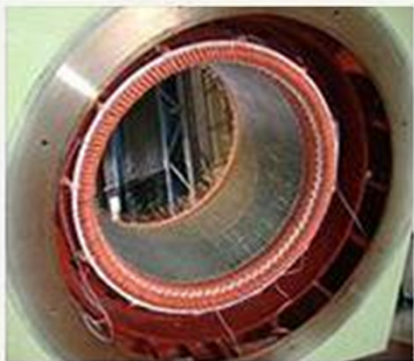
The non-connection end of the stator is shown, fully wound. The stator winding has been blocked and the end winding support applied.
