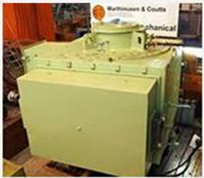
The completed motor is tested in the M&C large machines test bay at full voltage, i.e. 11000 V.
